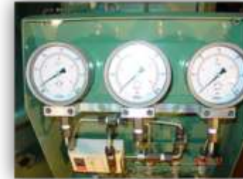
Pressure Gauges & Safety Controls
