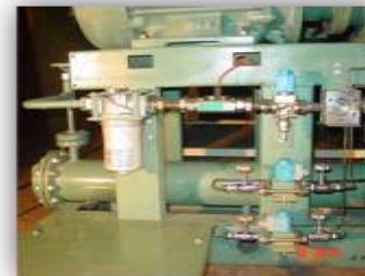
Lube-oil system & Oil Cooler
