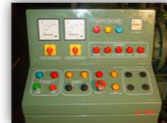
Screw Comp-unit Electric Panel
