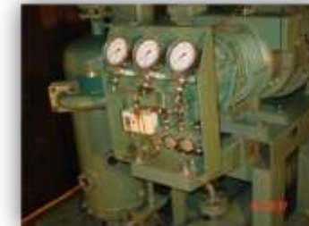
ICL-Bitzer Compressor Unit
